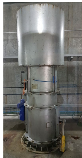
Figure 1: Capture chamber for an OWCs in Mutriku MOWC
